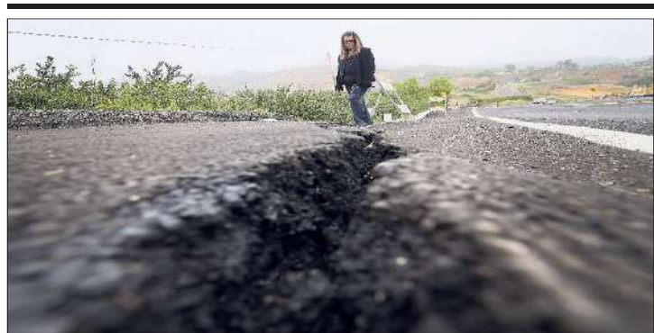
EVA ALBUJA surveys landslide damage near her Rancho Palos Verdes home. ALLEN J. SCHABEN LOS ANGELES TIMES
